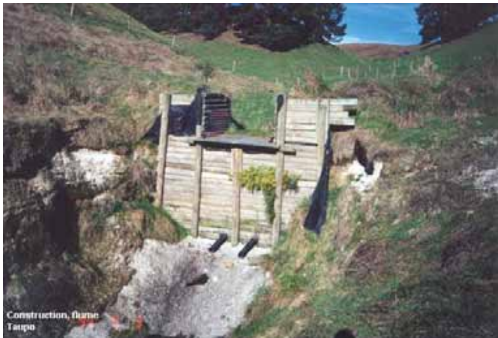
Photo 13: Flume designed to pass overland flow safely over the gully head without causing erosion.
