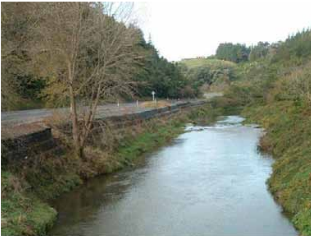
Photo 12: Gabion baskets used to protect a riverbank from erosion.
