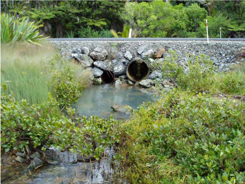
Figure 101: A recently installed road culvert along Whangapoua Road that is perched higher than the old culvert.
