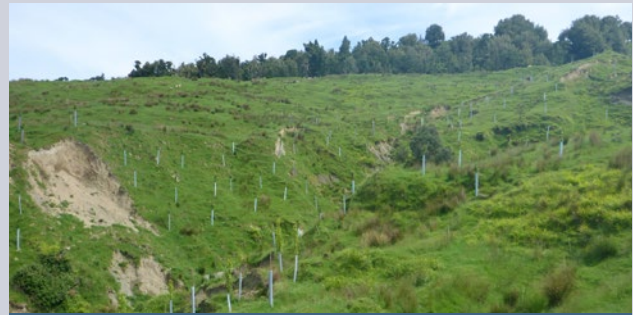
Pole planting on steep eroding hill country in the Lower Mokau catchment addresses mass land movement.
