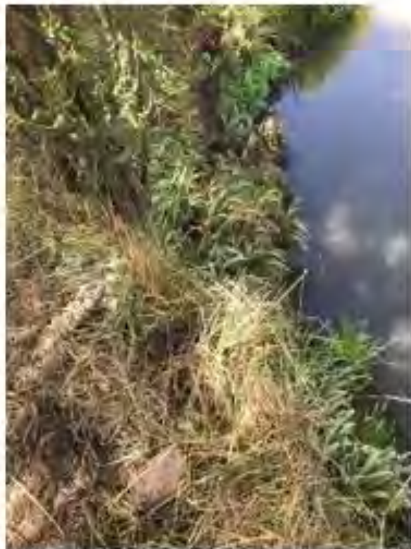
Photograph 2 Stream bank slumping reported by landowner to be caused by Koi Carp eroding the sediment beneath
