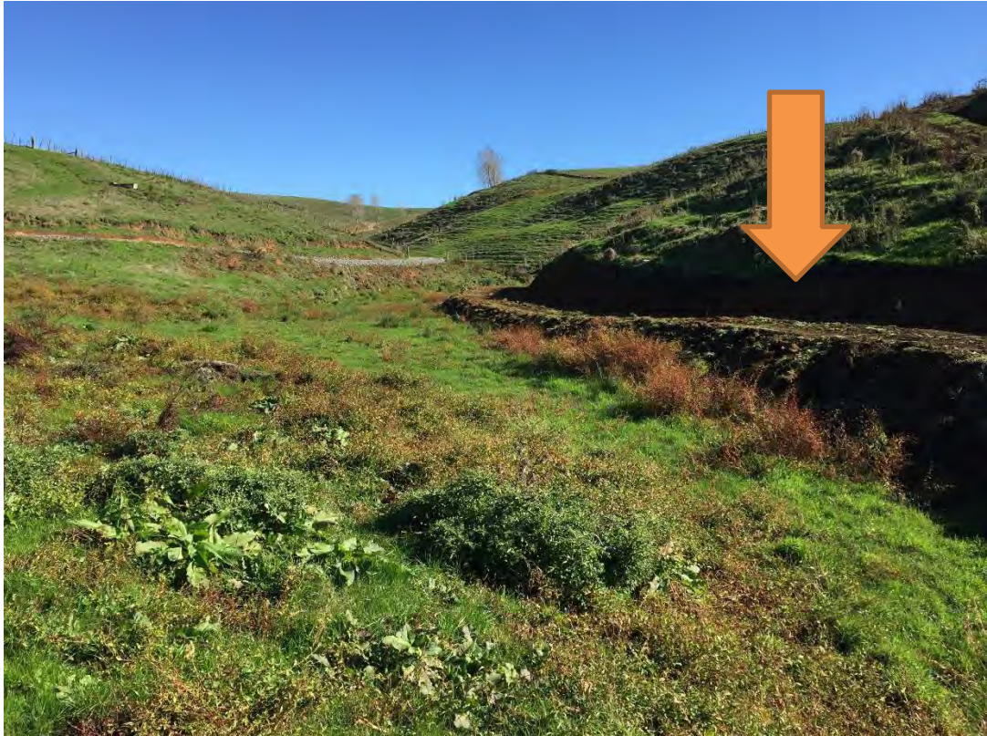
Figure 4: Photo of Farm 2 with earthworks preparation for fencing at a 1st order / ephemeral stream
